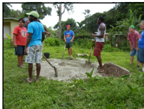
Mixing concrete. Glynn Roberts (center, red bandanna), Brian Hurlbut (green bandanna), Adam Nollsch .
